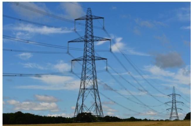
Additional electrical distribution may be required for AI data centre development
