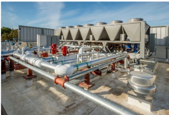
Data centre cooling system
